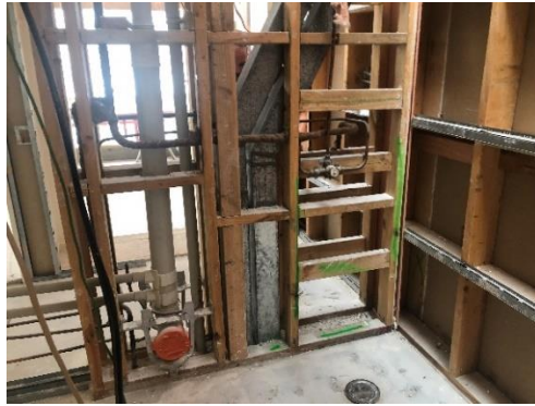
Bathroom IT walls prior to timber remediation
