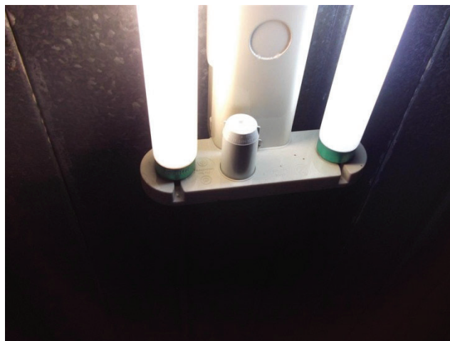
Figure 9 - Obsolete light fittings in Garages
