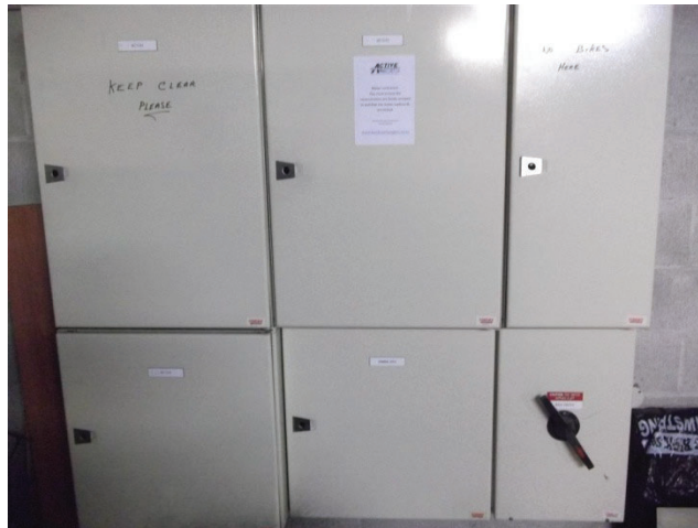
Figure 6 - Main building switchboard
