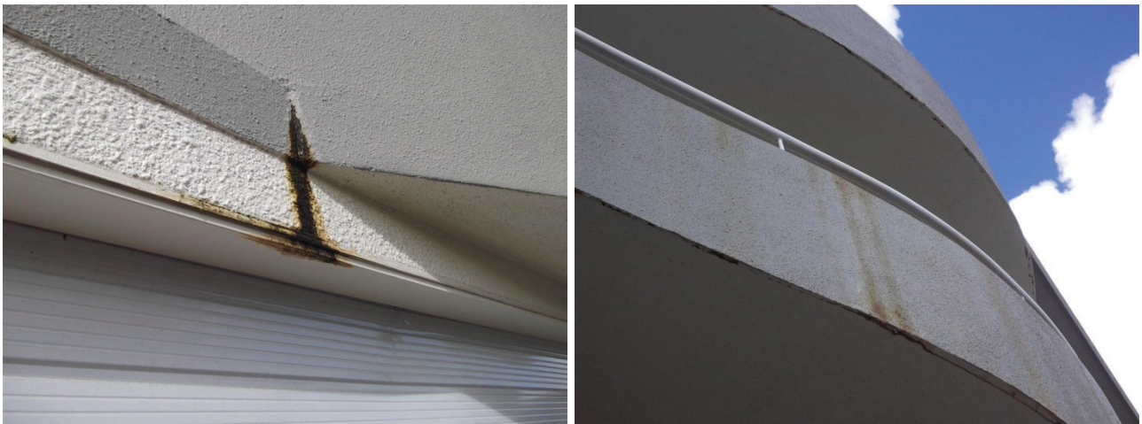
Figure 3 - Water ingress through decks
