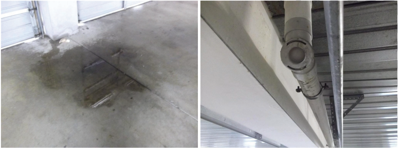
Figure 10 - Leaking pipework in Garage
