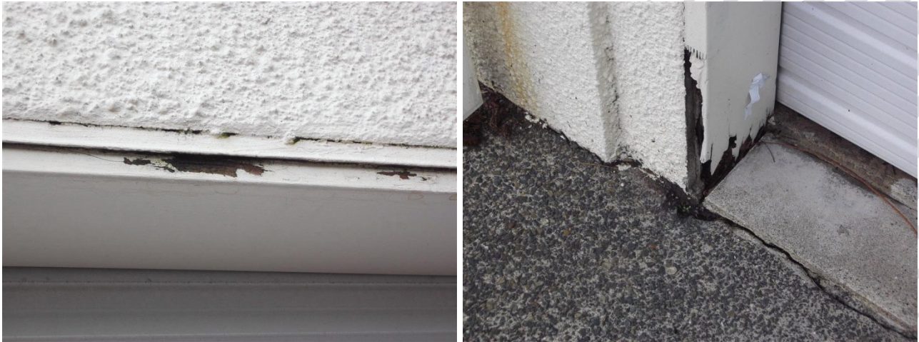
Figure 4 - Decay to Garage door sills
