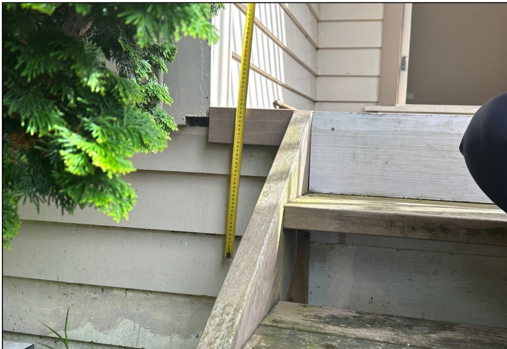
Figure 7: Site Investigation of the site after the impact of January Flood
